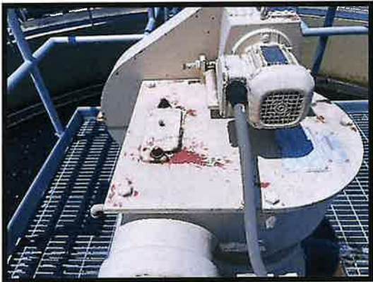
Figure No 11 – Peeling Topcoat Drive Motor
