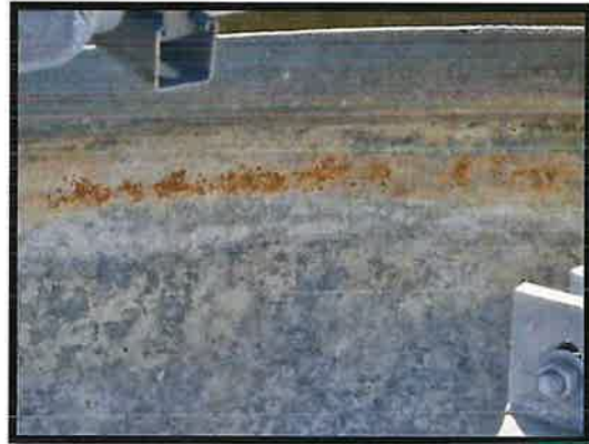
Figure No. 24 – Corrosion in the Stilling Well
