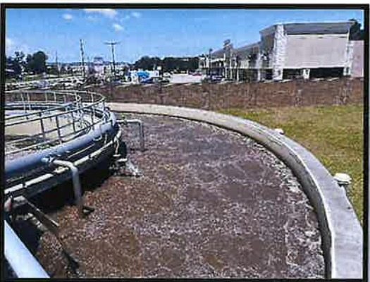
Figure No. 7 – Aeration Interior
