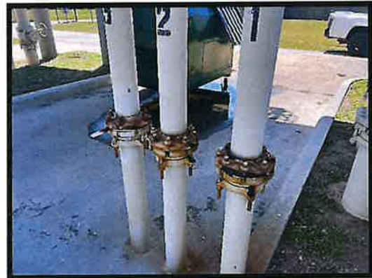
Figure No. 38 – Corrosion on Piping
