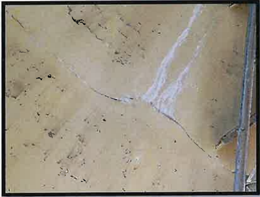
Figure No. 19 – Cracked Coating Clarifier Floor
