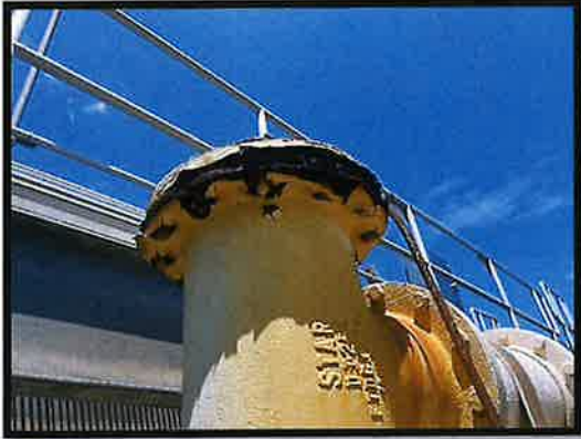
Figure No. 17 – Coating Failure with Corrosion Piping
