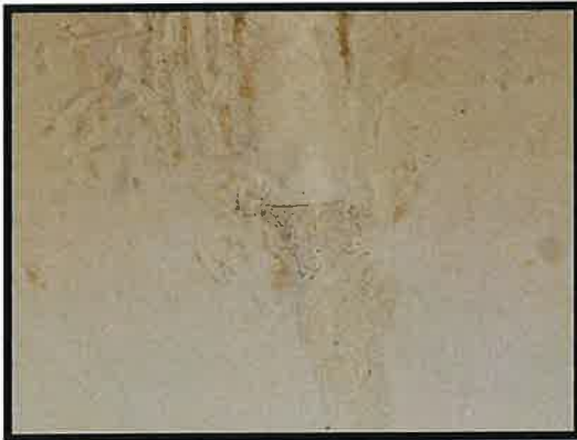
Figure No. 22 – Cracked Coating Clarifier Interior
