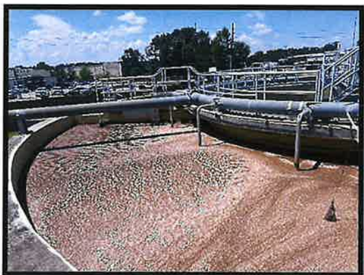
Figure No. 8 – Aeration Interior
