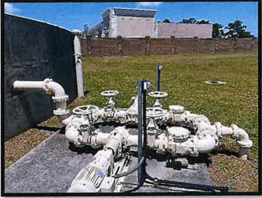
Figure No. 10 – Piping
