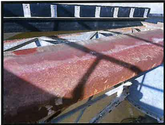
Figure No. 21 – Corrosion on Skimmer
