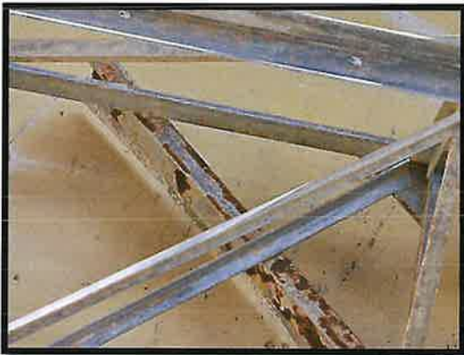
Figure No 25 – Corrosion on Scrapers Blades
