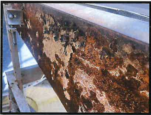
Figure No. 15 – Corrosion on Skimmer
