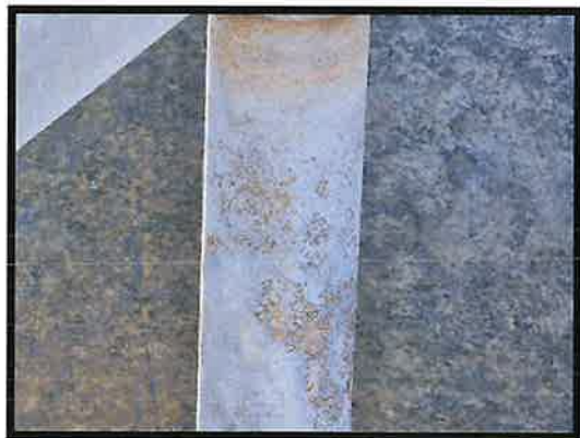
Figure No. 26 – Corrosion on Pipe in Stilling Well
