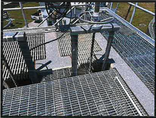
Figure No. 39 – Head Works Gates
