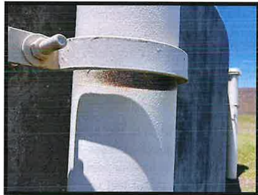
Figure No. 4 – Corrosion on Piping
