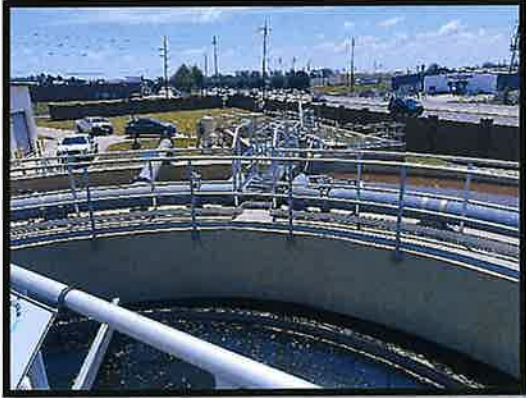
Figure No. 14 – Digester Interior
