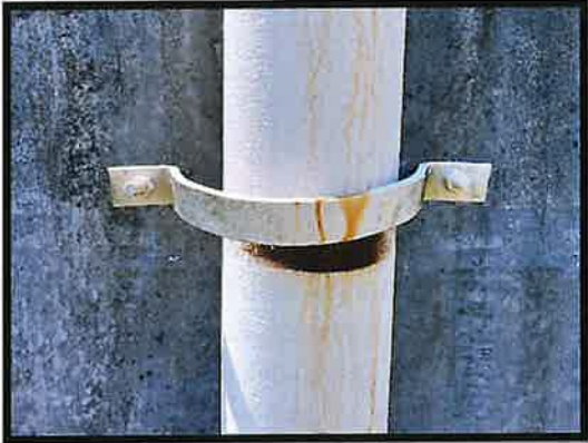
Figure No 9 – Corrosion on Piping
