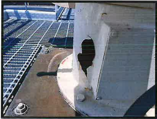
Figure No. 3 – Coating Chips with Corrosion Drive Motor
