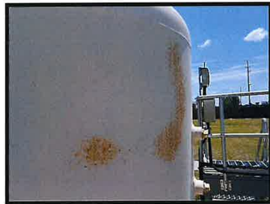
Figure No. 30 – Corrosion on Pressure Tank
