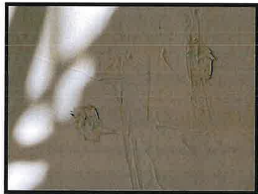
Figure No. 16 – Failed Area of Touch-up Coating
