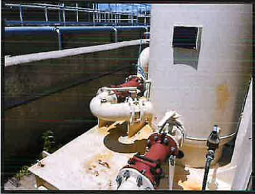
Figure No. 31 – Corrosion on Pressure Tank
