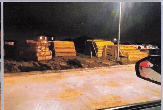
Hot water heater left in plan sight with box as well
